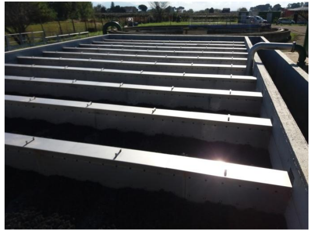
Figura 10. Vasca media clarifier.
